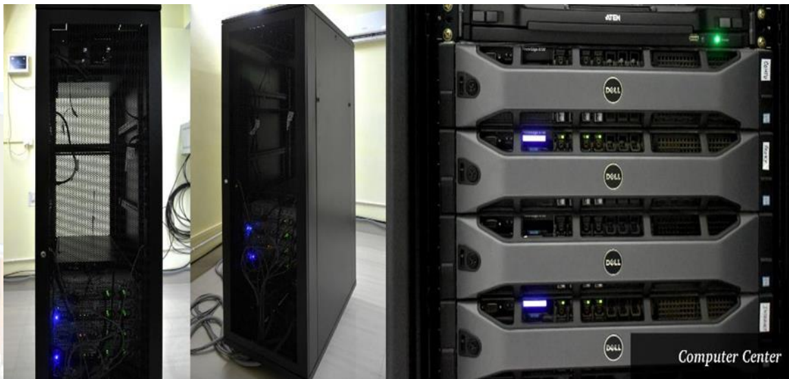
Figure 5: Server room at IIIT Bhagalpur
